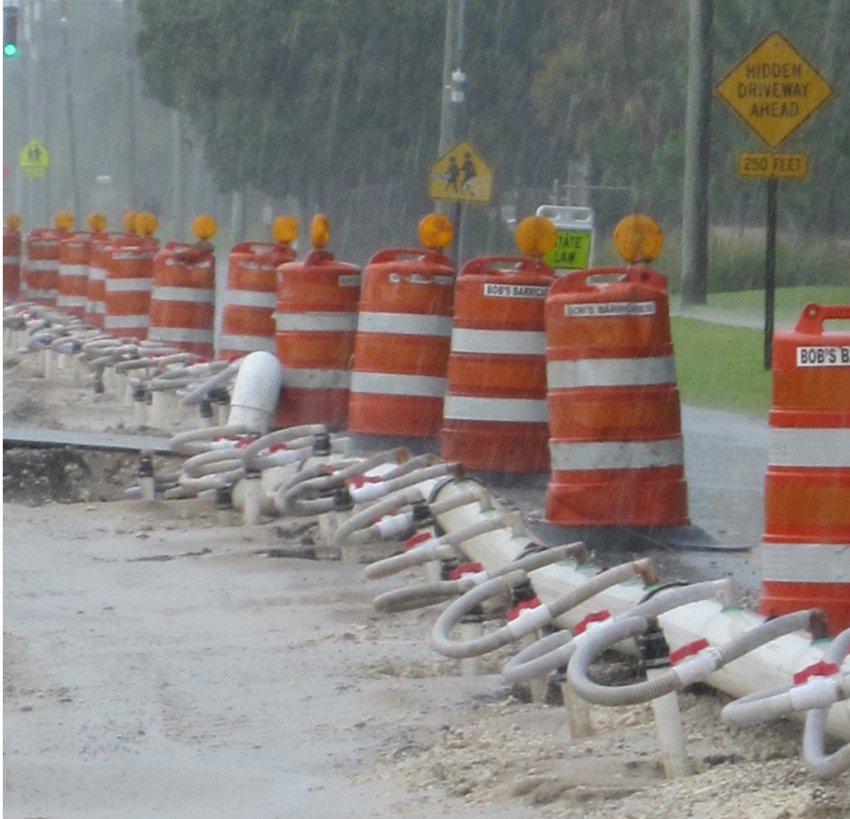
Figure 105. Well point system installation to help drain a roadway construction project in Town of Davie, FL
