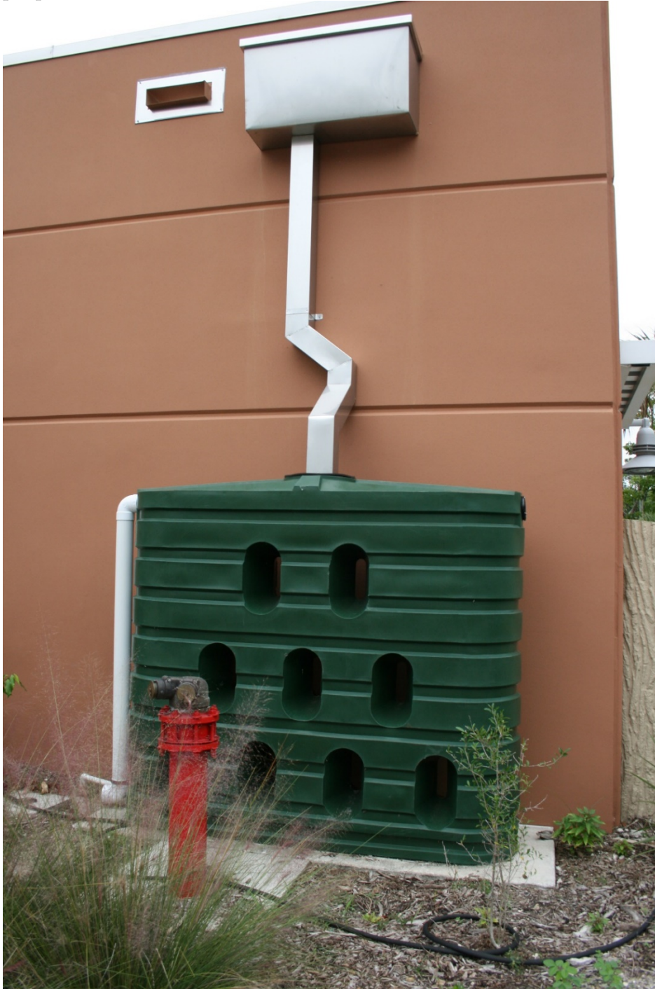
Figure 54. Rainwater harvesting cistern (used for irrigation) at the Pine Jog Environmental Center in West Palm Beach, FL
